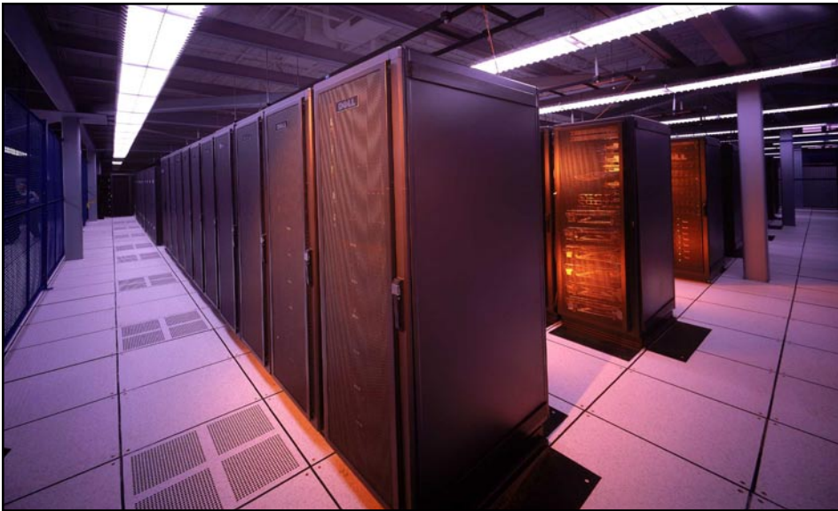
Inside the Herakles Data Center, the newest generation of servers housed there are more powerful and more compact than ever, producing more heat and more cooling capacity demand.
